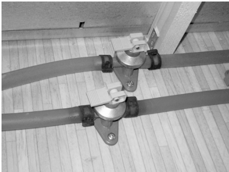
Fig. 158: Closed drain valves
