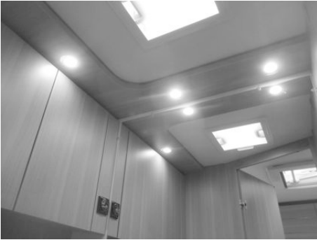
Fig. 54: Bathroom lighting, example
