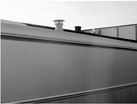
Fig. 95: Exhaust gas stack of the gas heater
