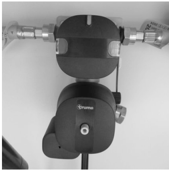
Fig. 89: Gas supply (with Eis-Ex and remote control)
