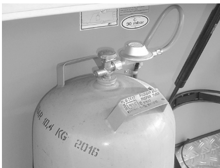
Fig. 112: Gas bottle with pressure reducing valve
